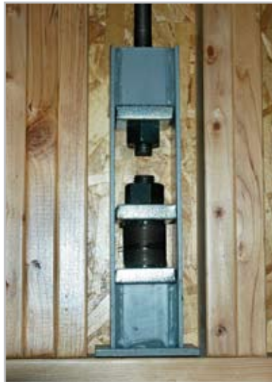
Previous Anchor Tiedown System
