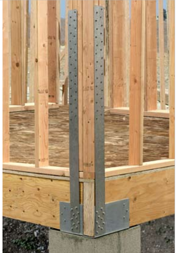
Typical ECCLQM Installation
