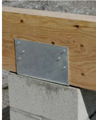
Typical CCQM Installation
