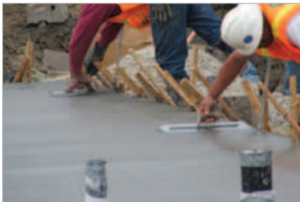
Eliminating bolts results in a slab that is flatter and easier to finish.
