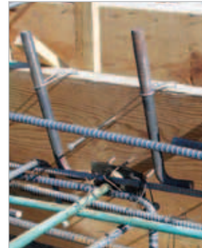
Hanging bolts on forms before the pour takes time and creates an opportunity for error.
