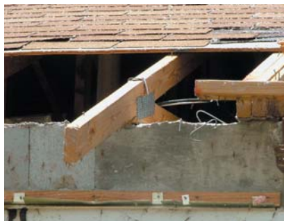
An example of some of the damage from Hurricane Charley.
