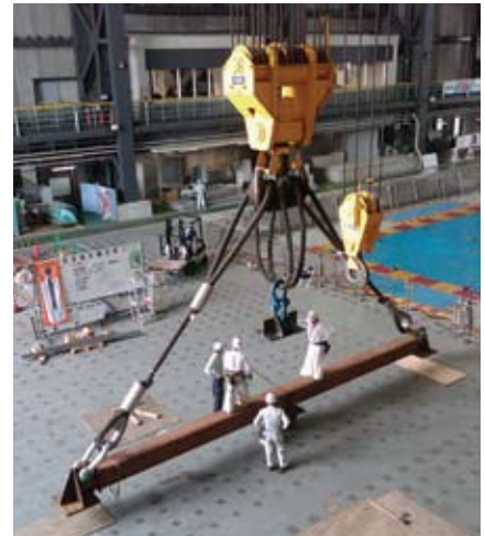
The 7-story structure was built on the lab floor and then had to be lifted onto the shake table using two 400 metric ton overhead cranes.
