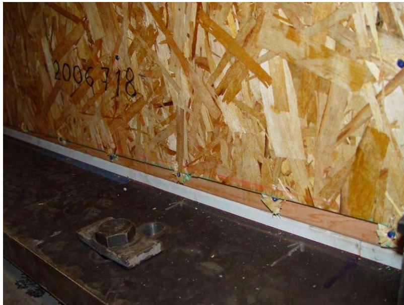
Figure 8 - Typical Sheathing Nail Tear-Out.
