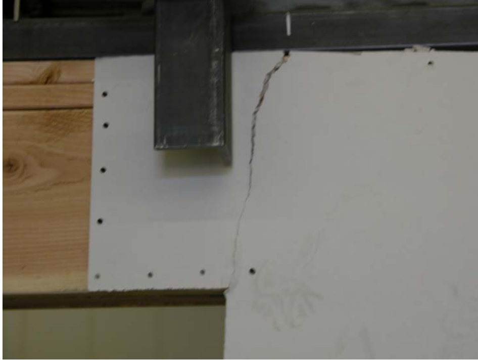
Figure 8. Typical Initial Failure of 4_1 Wall Specimens – Cracking of Gypsum Wallboard (shown near top of specimen).
