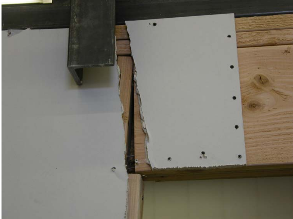
Figure 10. Continued Failure of 4_1 Wall Frame Specimens – Further Opening of Cracks in Gypsum.
